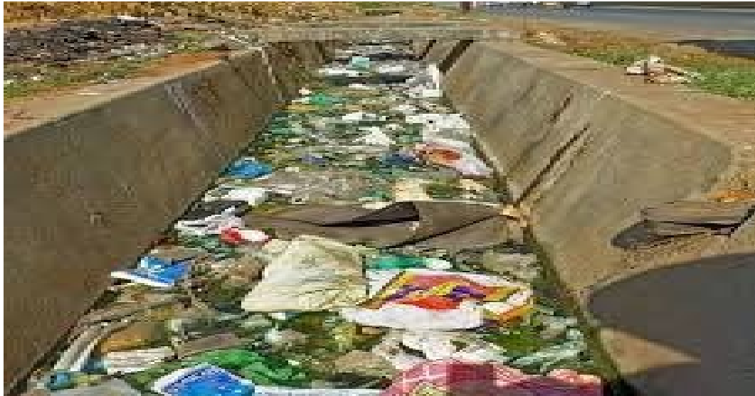
Fig. 5: Solid waste blocking drains
