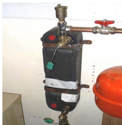
Figure 14: Shows the heat exchanger
