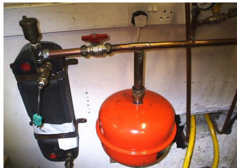
Figure 16: Shows the connections of the heat exchanger and expansion valve
