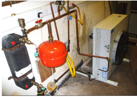
Figure 15: Shows the connections of the heat exchanger, water pump, heat rejection fan and expansion valve
